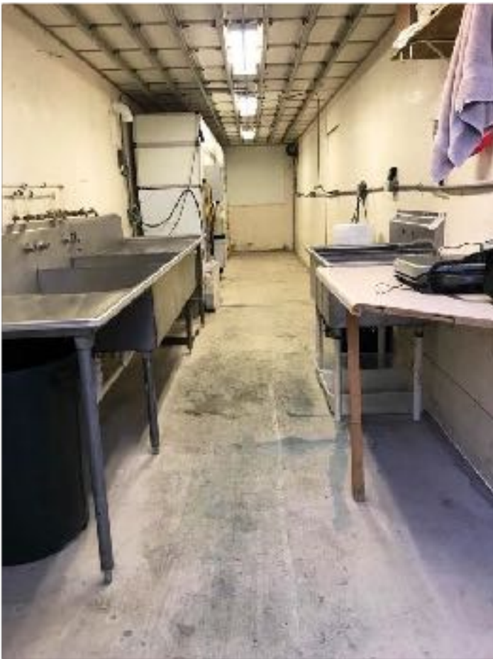
Commercial Kitchen in Trailer
